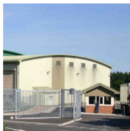
Poor elevational design, with vents staining the facade
