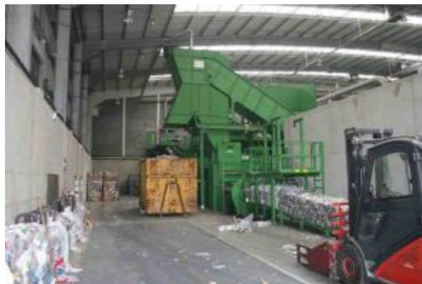
Bulking up facilities within a MRF
